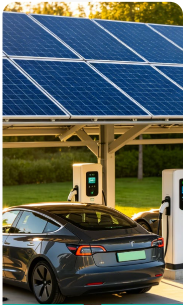
EV Charging Station
